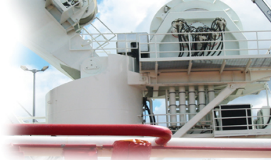
↗ Complete stripping of hydraulic pipework and replacing with new, for large supply vessel.
